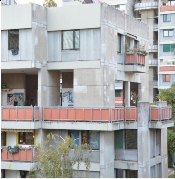
Fig. 9: Traces of repair works on the concrete façade of house no. 31.
